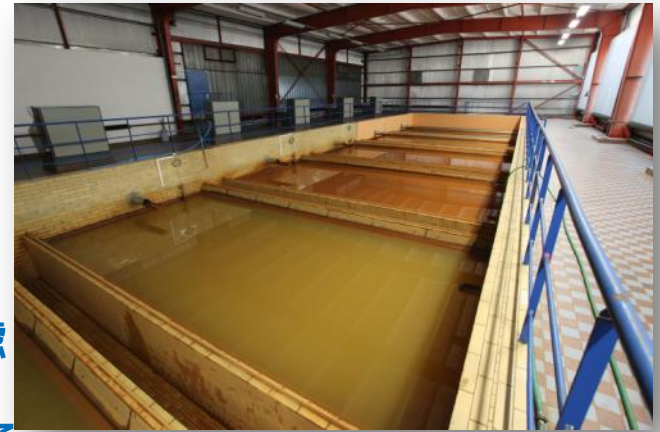
Copyright: Iron/ Manganese removal plant, Wikipedia, Petr Novák
